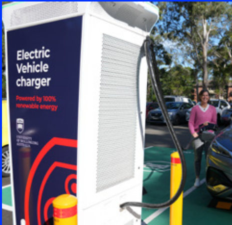
EV CHARGING STATIONS INSTALLED IN 2024
